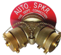
Fire Department Siamese Connection
